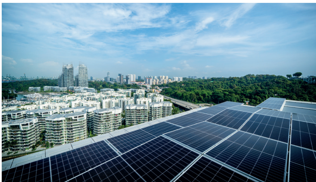
Seven properties within Keppel REIT's portfolio, including Keppel Bay Tower in Singapore, are fully powered by renewable energy.
